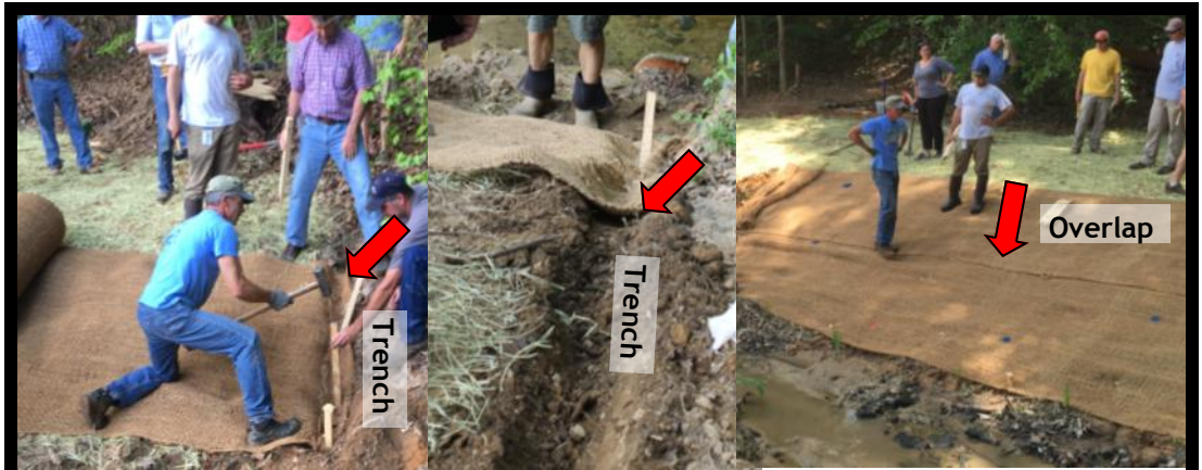
Matting 1) Lay start of matting in trench and tamp in 2' oak stakes with nail on end. Add every 1.5' to top of trench. Overlap extra matting rolls by 1'.
