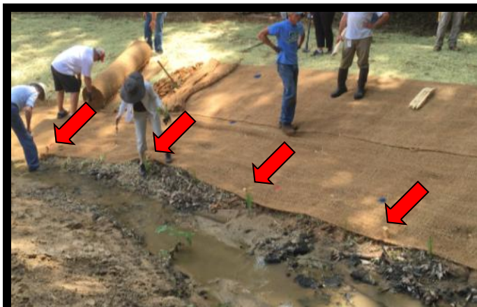
Matting 2) Roll out matting and tamp down oak stakes every 4' at water's edge. Follow the contours of streambank with matting constantly touching soil. Do not pull taut.
