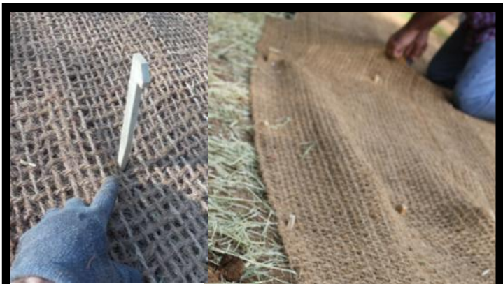
Matting 3) Add 2' oak stakes every 10' to top of matting. Randomly hammer in eco-stakes every 4'-6' feet throughout the matting as well as along the top edge.
