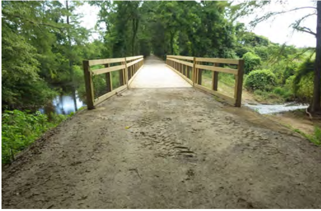
Example of a rehabilitated railroad bridge on the Arkansas Delta Heritage Trail (led by Alta)
