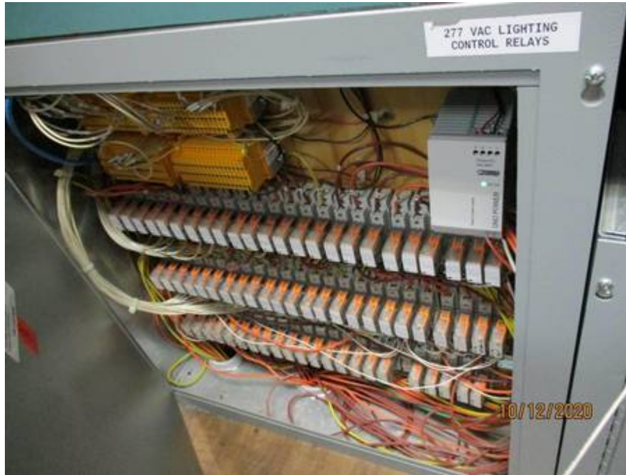
Figure 13 — Lighting Controls in Central Control (typical of lighting and phone controls)
