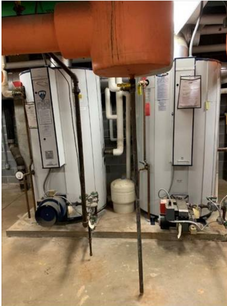
Figure 5 – PVI Hot Water Boilers in Courthouse serving the Detention Center
