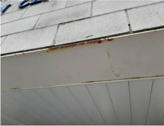
Figure 2 – Example of rust at lintel
