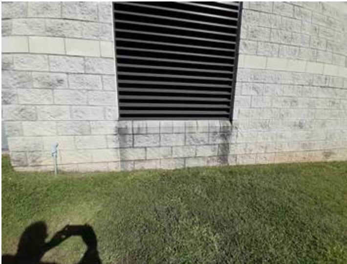
Figure 5– Mold and mildew on exterior walls (louver at vehicular sallyport)
