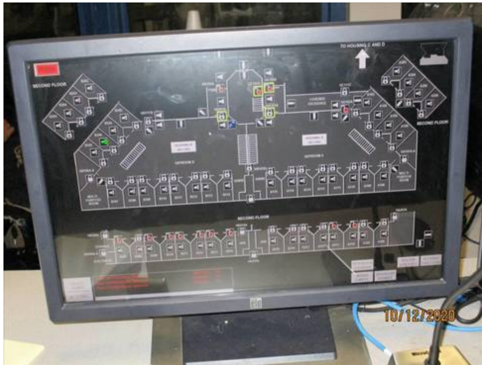
Figure 12 — Touch screen control panel (work station) in control rooms (typical)
