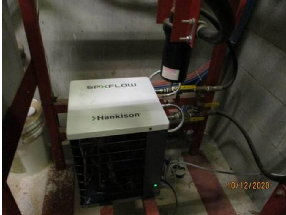
Figure 5 — Locking Pneumatic Air system refrigerant dryer
