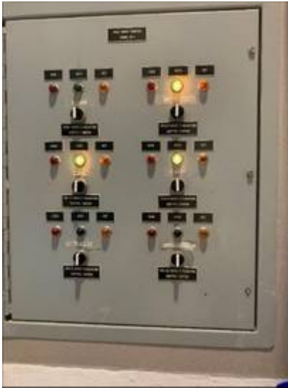
Figure 3 – Smoke Control Panel
