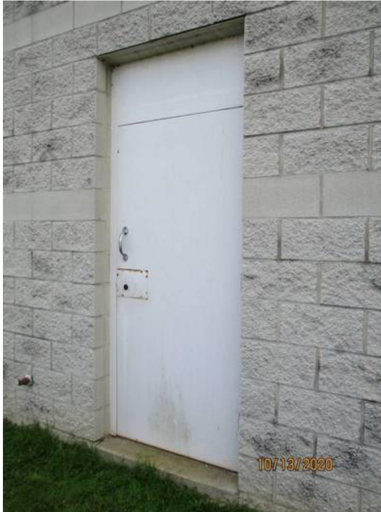
Figure 3 — Security Hollow Metal Door with mechanical hardware (Equipment Room)
