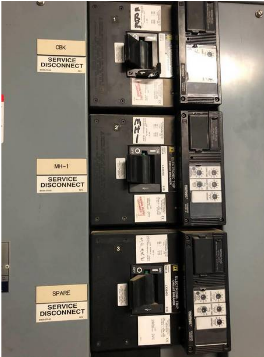
Figure 8 – Mislabeled panelboards in main electrical room
