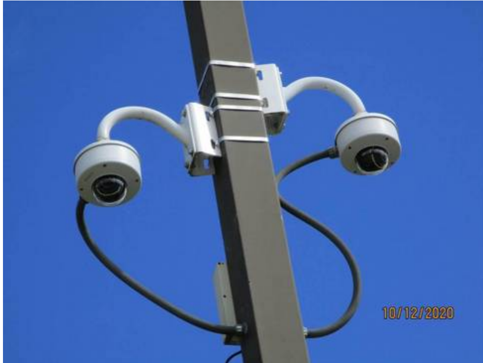
Figure 22— Pole mounted IP-CCTV Cameras (typical)
