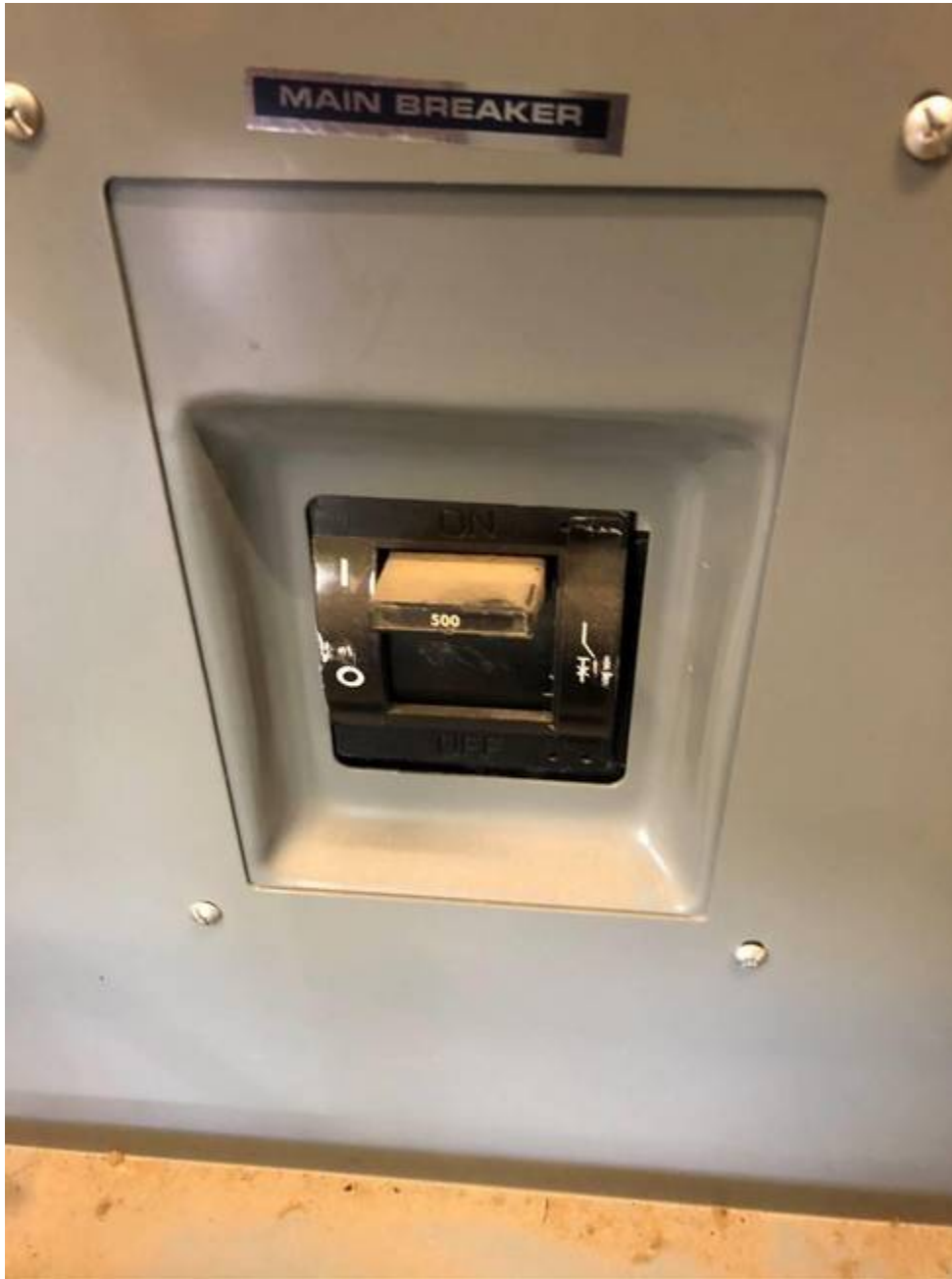
Figure 4 — 500amp main breaker for Main Service Distribution Panel EH1
