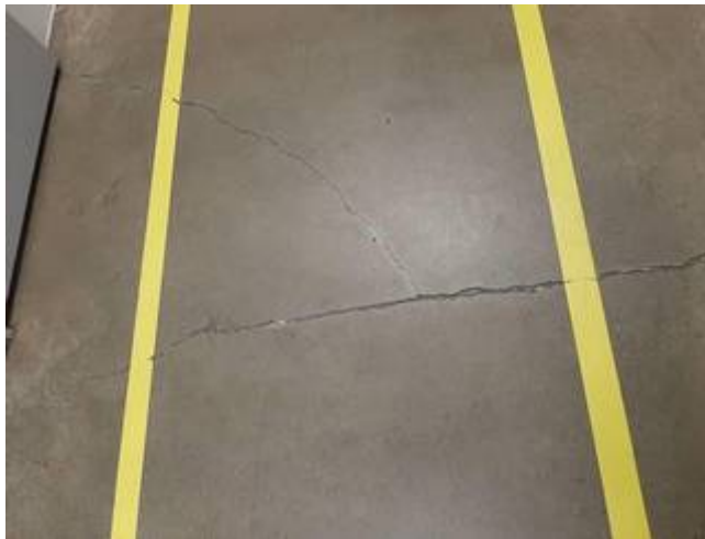
Figure 1 – Example of cracking observed in concrete floor slab.
