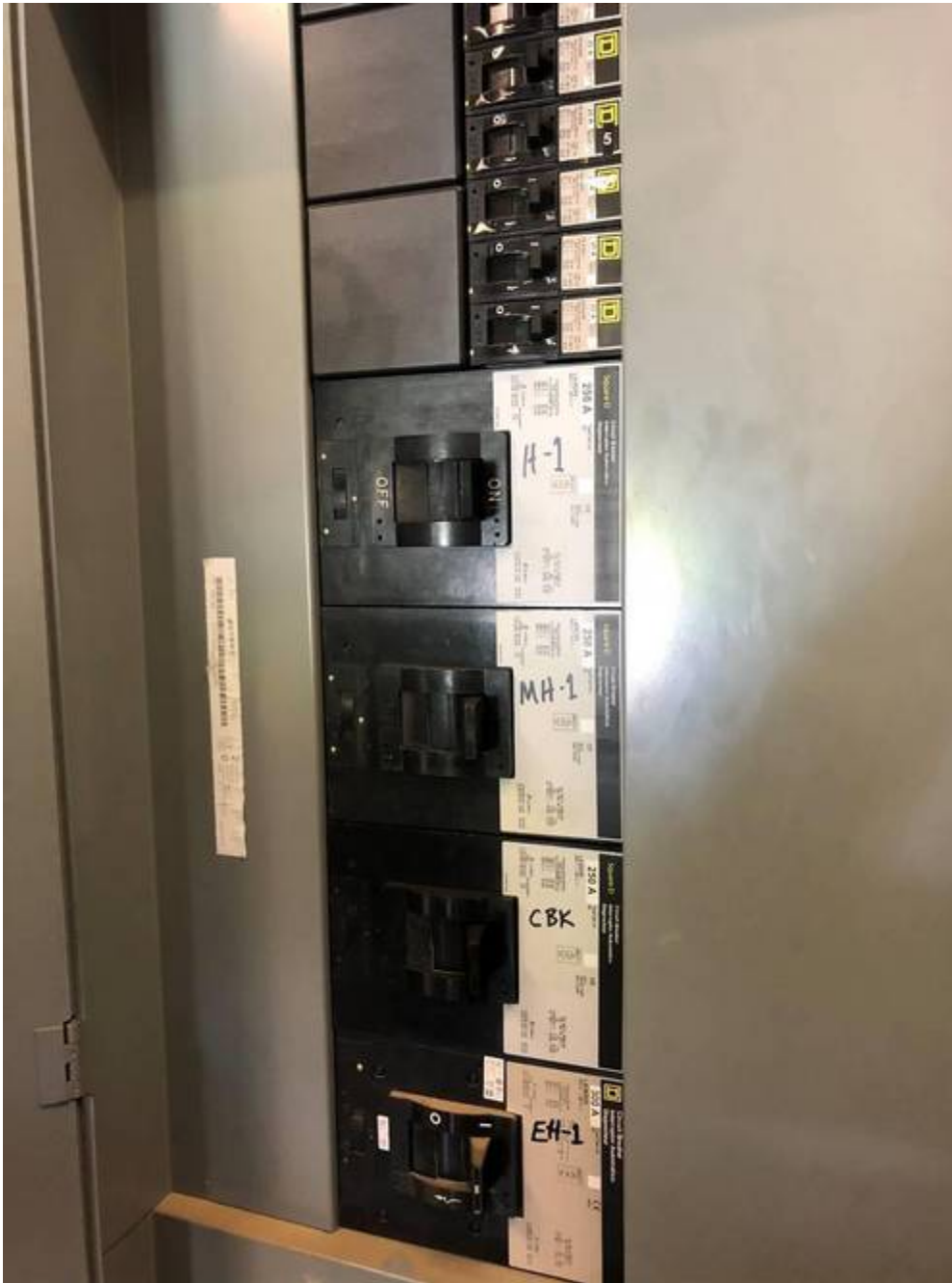
Figure 3 — Main Service Distribution Panel EH1
