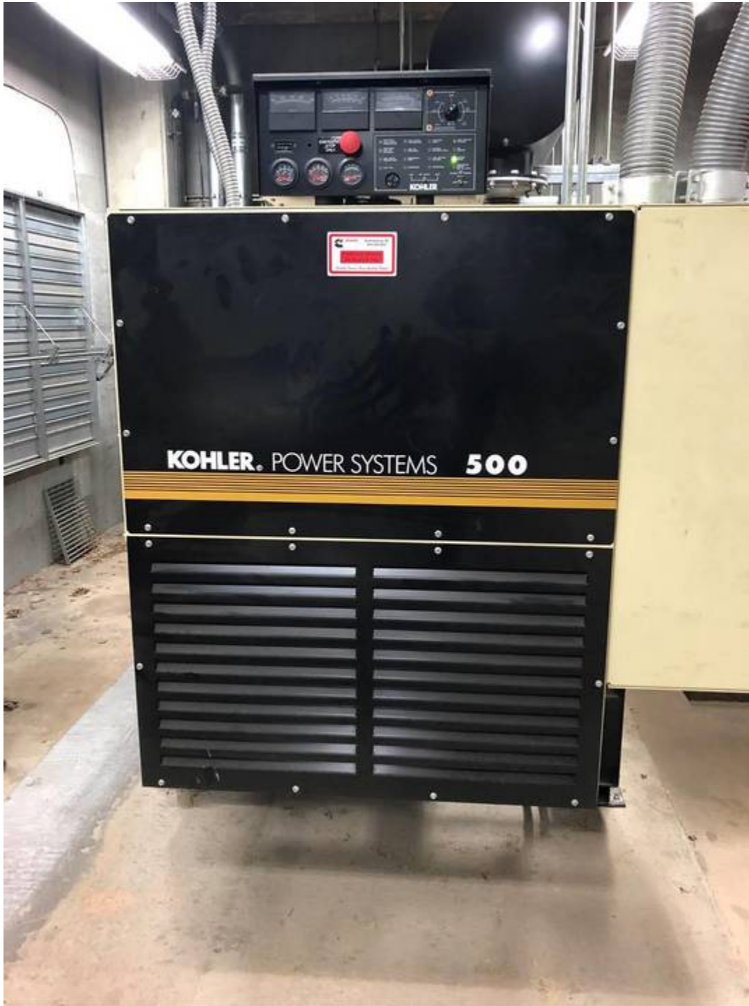
Figure 5 — 500kW Emergency Generator located in Courthouse
