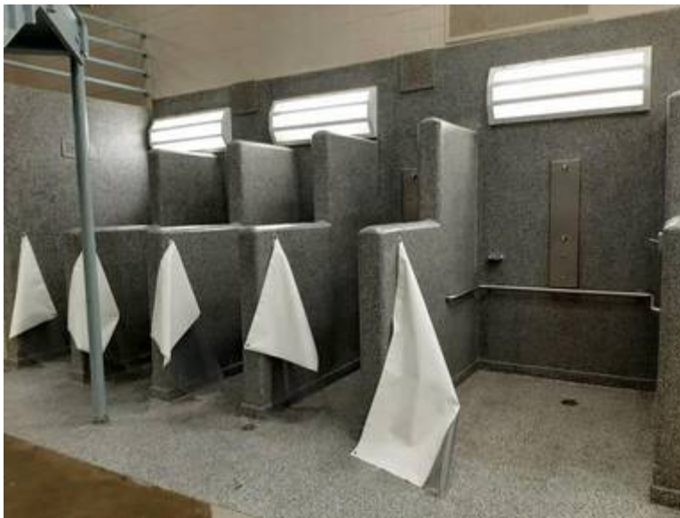
Figure 12 – Coating at inmate showers.
