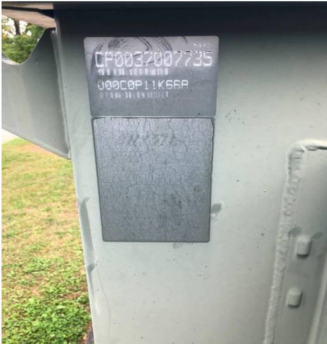
Figure 1 — 500kVA Utility Transformer that supplies power to the facility
