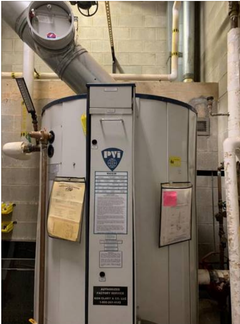
Figure 6 – PVI Hot Water boiler serving Kitchen and Laundry in the Detention Center
