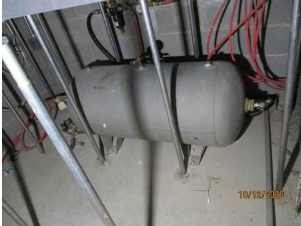
Figure 7— Locking Pneumatic Air System Emergency Reserve tank
