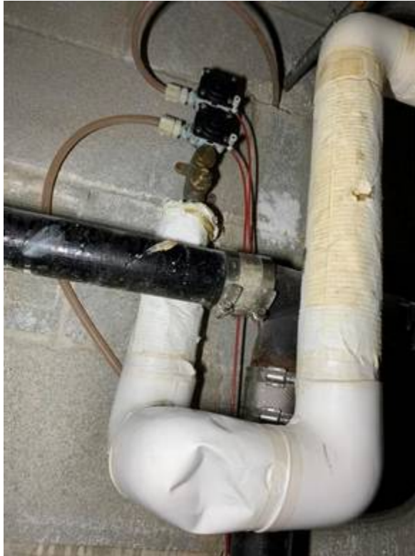
Figure 8 – Pneumatic Water Control Valves, Plumbing Chase
