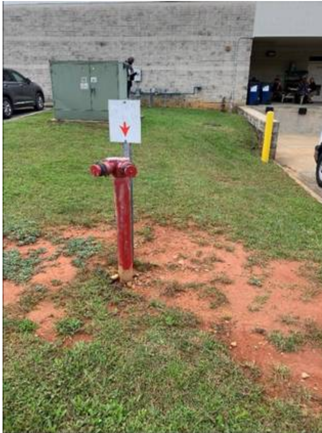
Figure 11 – Fire Department connection
