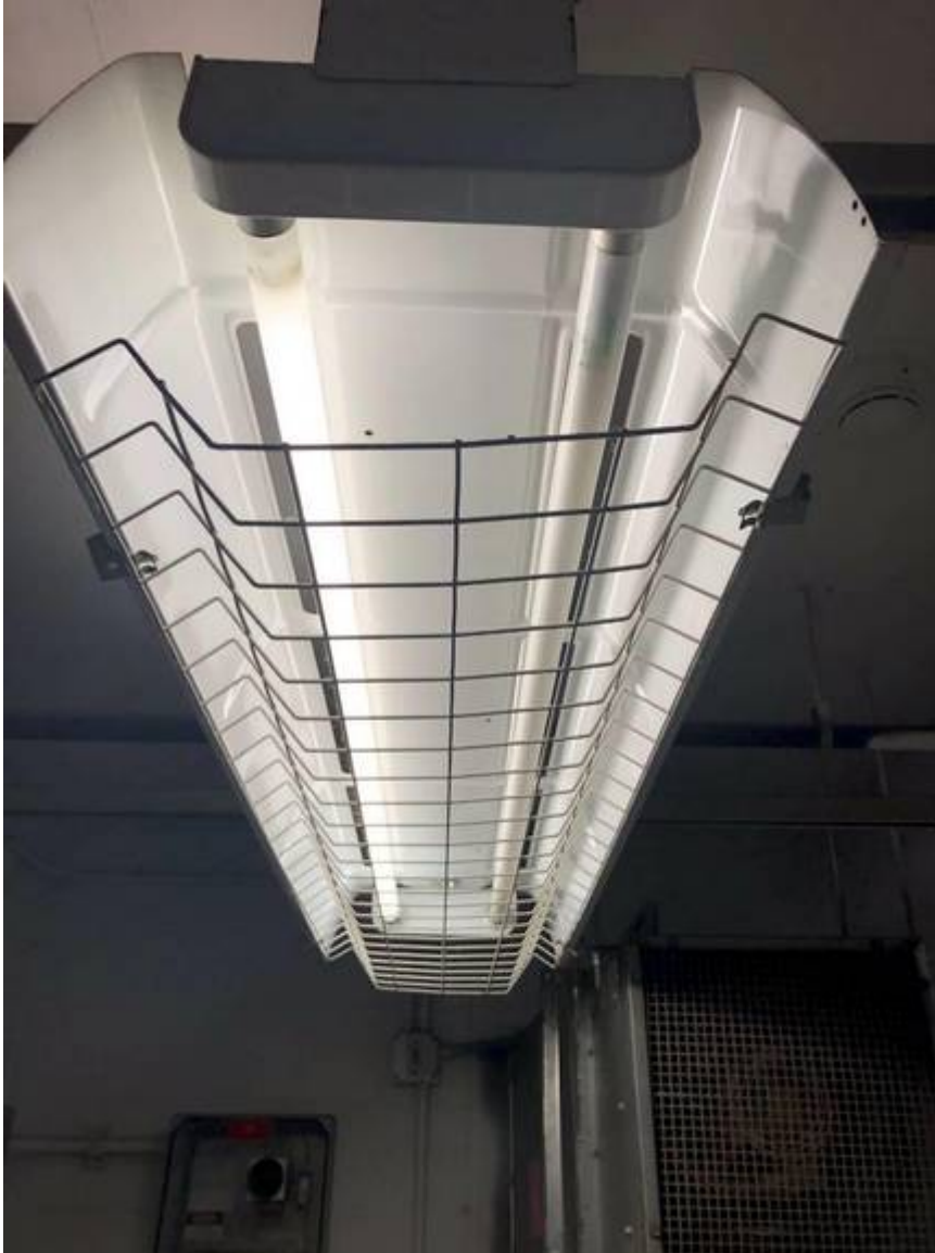
Figure 9 – Lamp replacement needed in several fixtures
