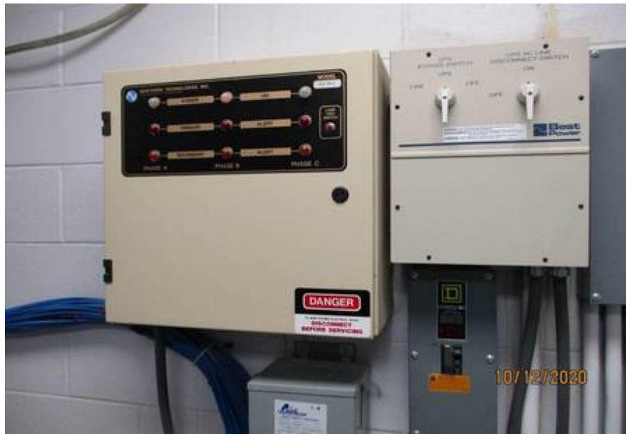
Figure 14 — Northern Technologies Surge Protection Device
