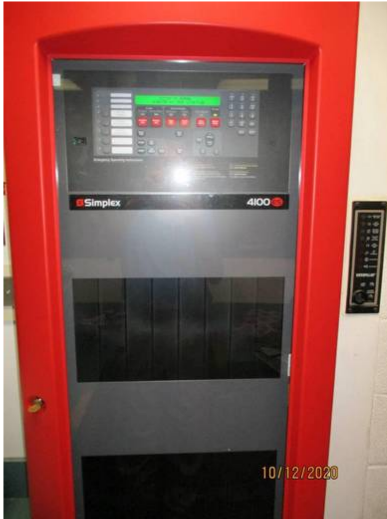
Figure 9 — Simplex 4100 Fire Alarm Panel in Central Control Room
