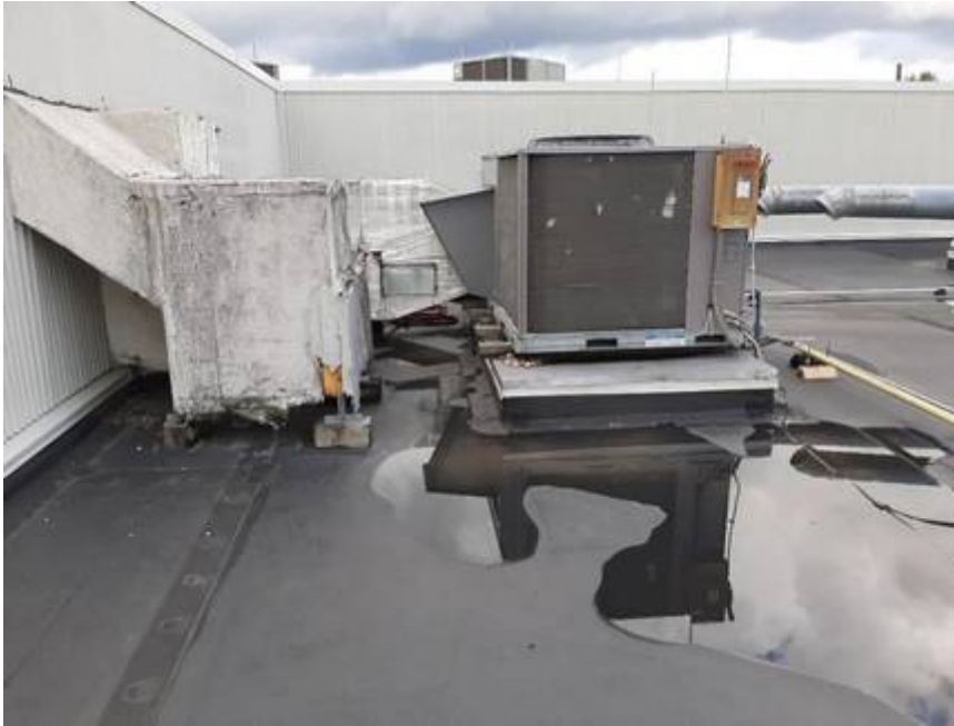
Figure 2 - RTU 5 – Insulation and Exposed ductwork
