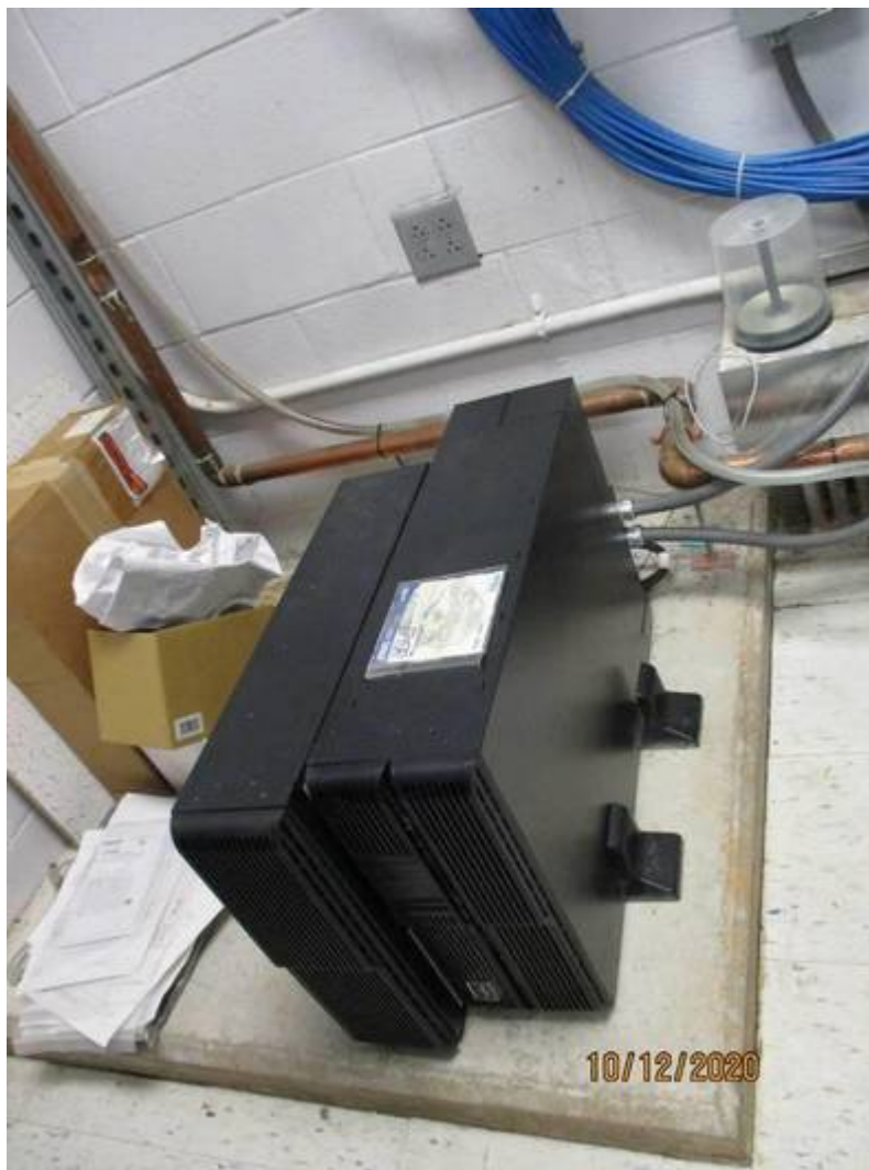
Figure 16 — Emerson UPS in Security Electronics Equipment Room
