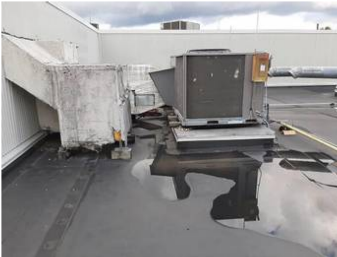
Figure 3 – Roof at support area-Equipment drainage
