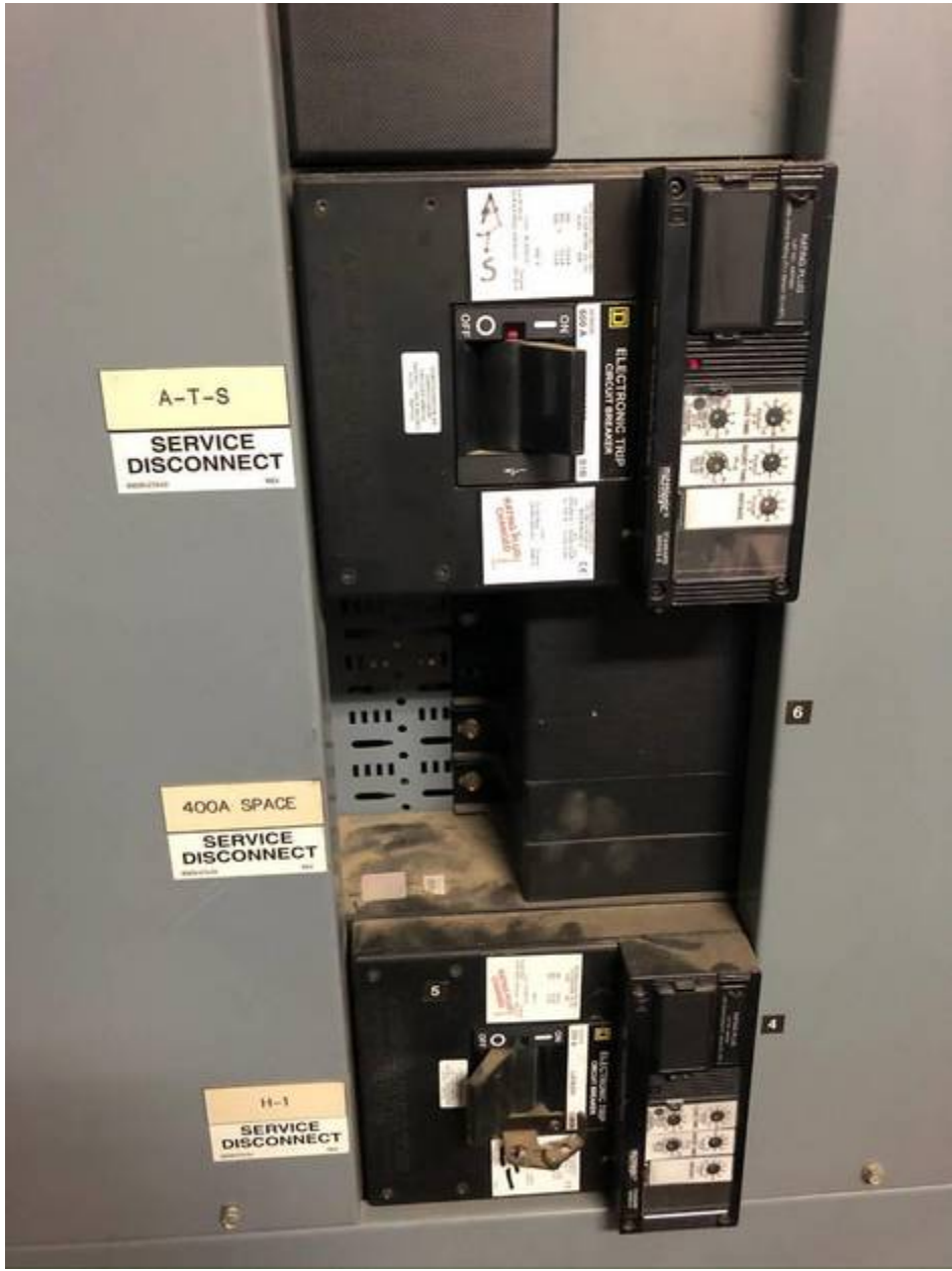
Figure 7 – Mislabeled panelboards in main electrical room
