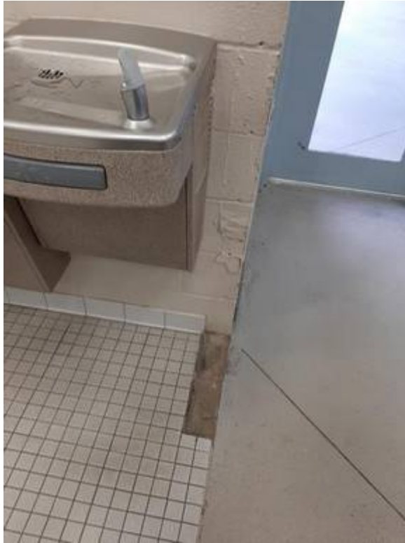
Figure 10 – Broken ceramic floor tile.
