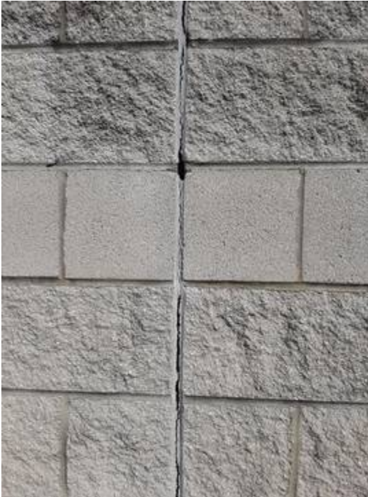
Figure 4– Caulking failure at masonry control joint
