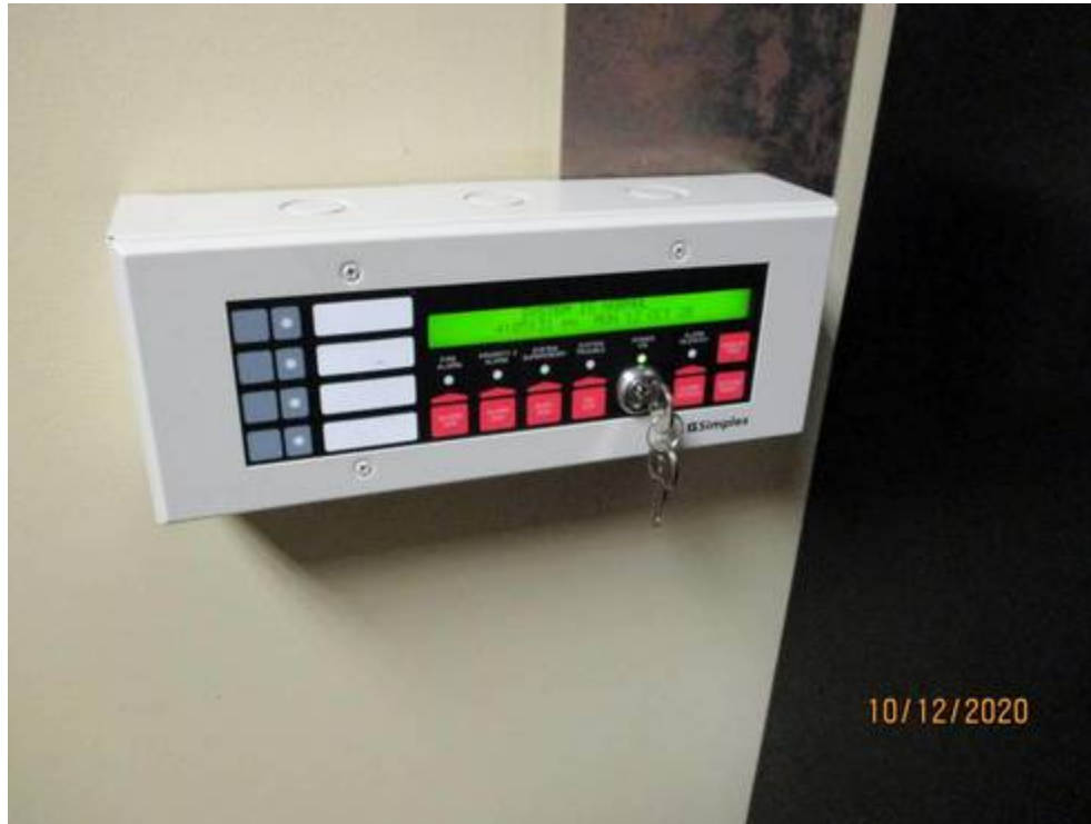
Figure 10 – Fire Alarm System Remote Annunciator Panel (typical)
