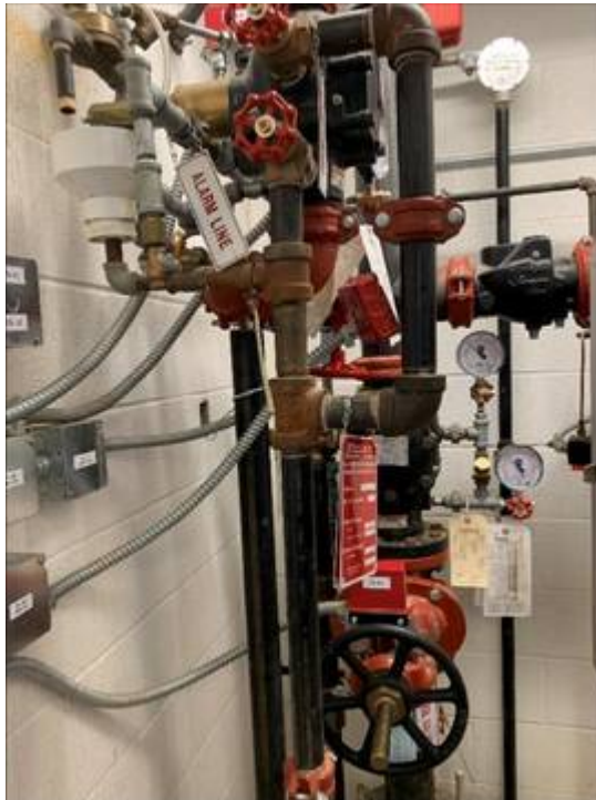
Figure 9 – Fire Protection Riser Main
