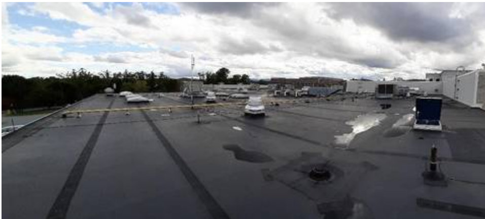
Figure 4 – Mechanical Roof Top Units
