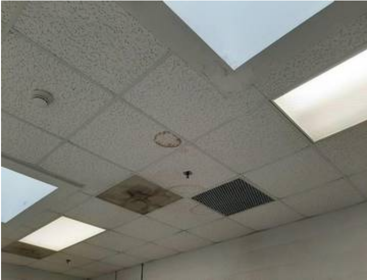
Figure 6– Water damage at ceiling tile; work release.
