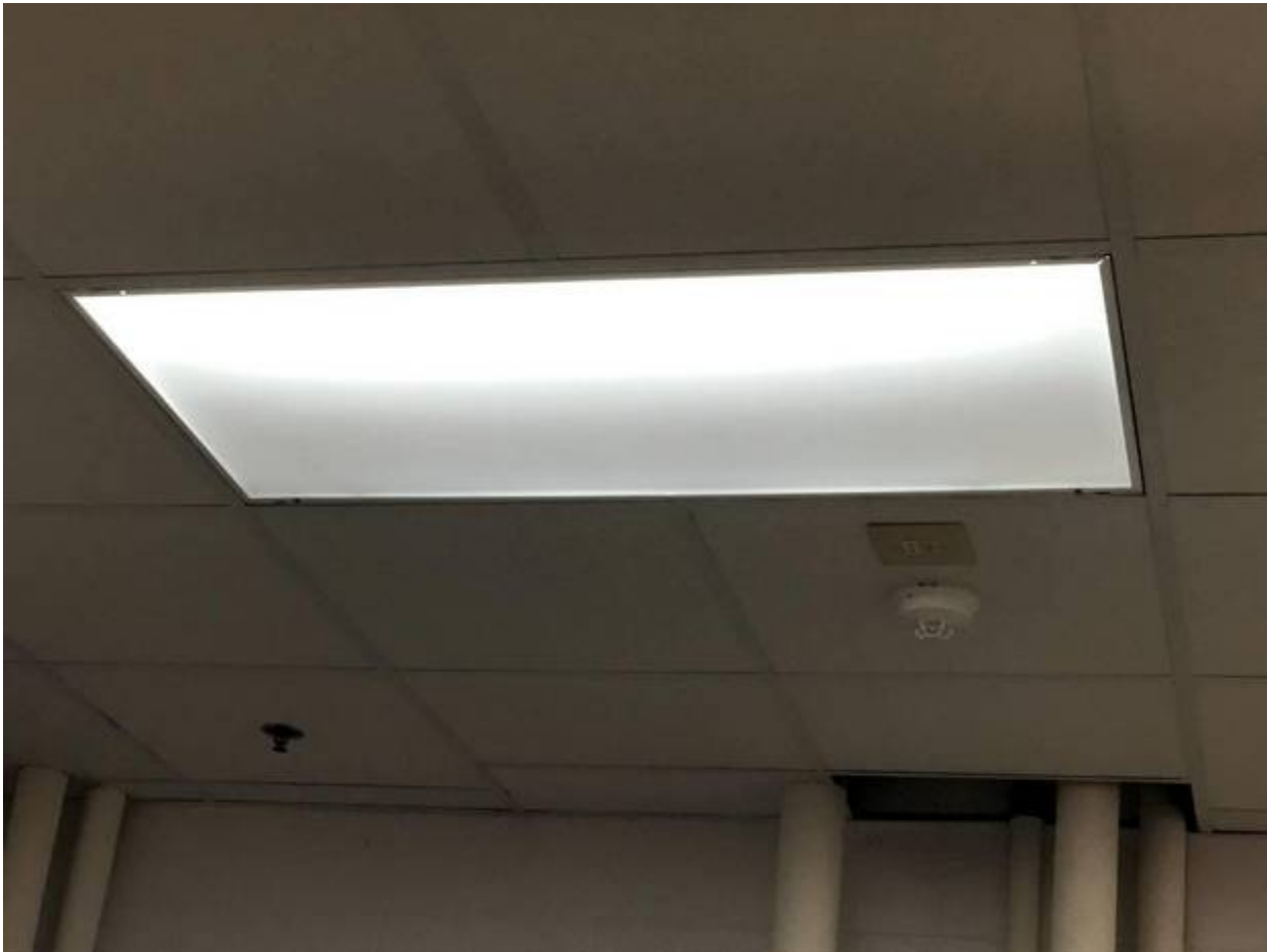
Figure 10 — Lamp replacement needed in several fixtures
