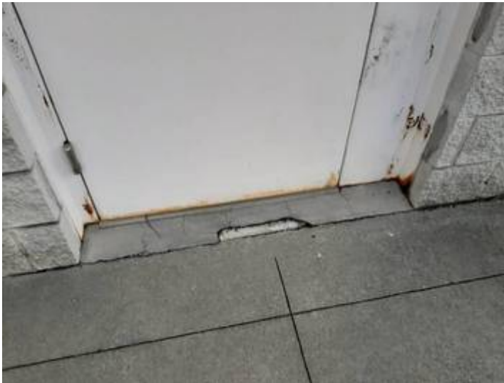
Figure 7– Rust at exterior doors and frames.
