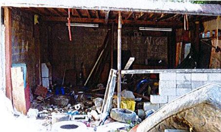
Building will be demolished because roof is falling
