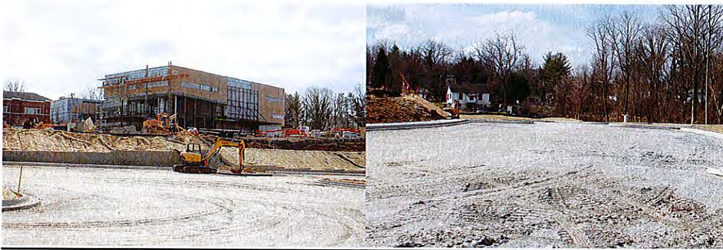
Site of the over-flow parking lot an endeavor independently made by Pardee.
