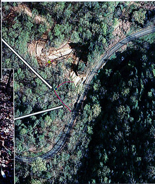
U.S. 64 Bat Cave Active Cut Slope Failure
