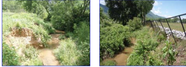
Severe Bank Erosion on Mud Creek
