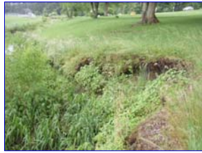
Erosion on Mill Pond Creek Bank
